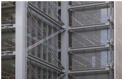
Figure 2: By introducing several load paths in the cantilevered framing lines, the exterior steel can be exposed.
